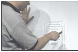
Tape the template to the desired area. Cut the drywall for the selected model.
